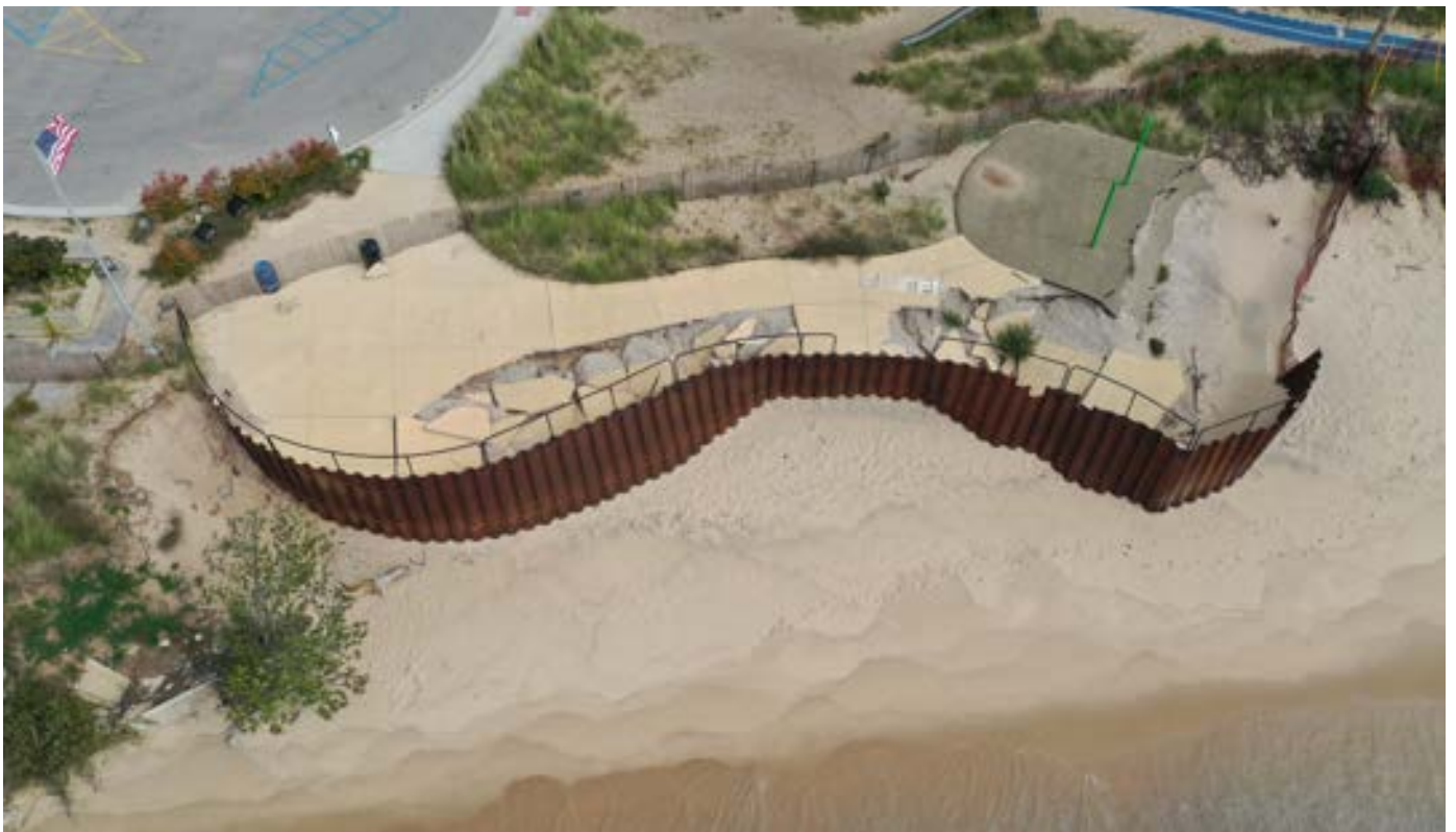
Image 2: Existing Sheet Pile Wall and Broken Paving
